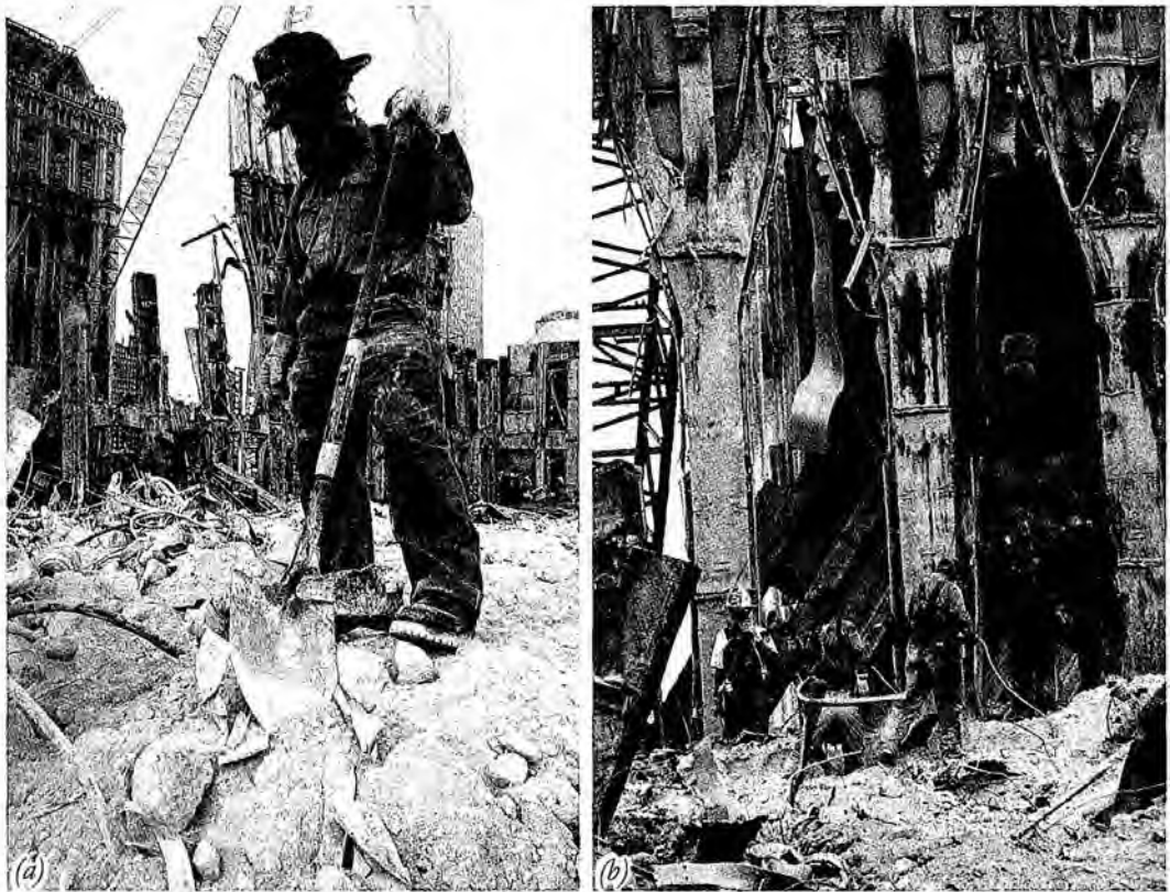
Figure 143. (9/13101) (a) Scooping up the building (b) Workers walk in thick dust atop the rubble pile, hardly higher than the lobby level
