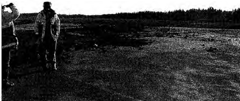
Figure 111. Pavement dislodged during a high-power engine run-up. 54
