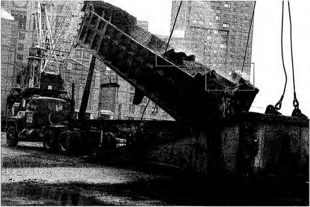
Figure 341. (3/15/02) A truckload of fuming dirt is sprinkled with water while being dumped. The yellow plattform then transferred the contents to a waiting barge on the Hudson River (at right). Enlargements of the two boxed-in regions are shown in Figure 342.
