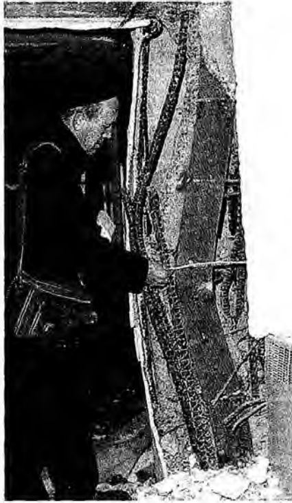
Figure 494. A buckled column, from the 1964 Alaska earthquake. This image is useful not only for illustrating buckling in general, but also the effects of support restraint.
