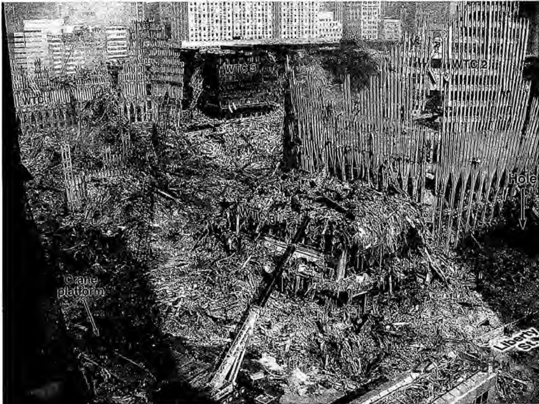
Figure 484. (9/22/01) These last standing columns are not buckled. Note the hole on the far right.
