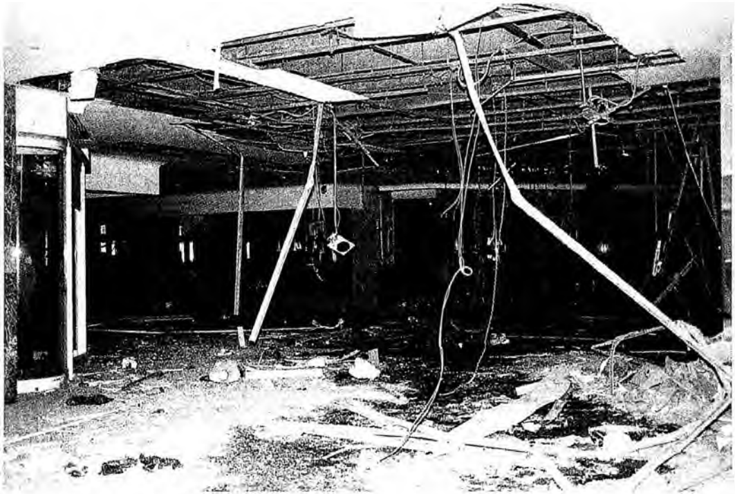
Figure 182. (post 9/11/01) What remains of the Strawberry store, viewed from Warner Brothers. 15 (Location A in Figure 183)
