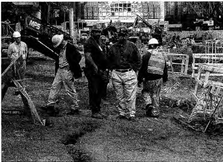
Figure 47. (10/10/01 ) Damage from earth-moving equipment along Liberty Street,
