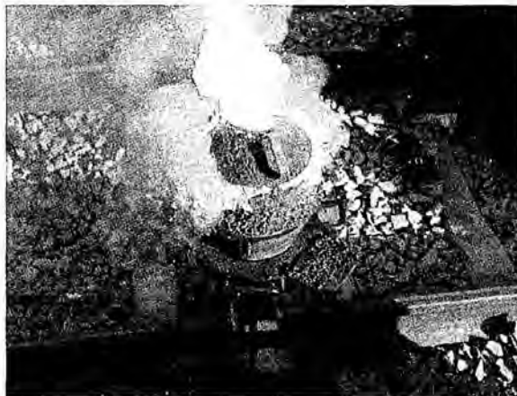
Figure 118. Thermite reaction proceeding for a railway welding. Shortly after this, the liquid iron flows into the mould around the rail gap. http://upload.wikimedia.org/wikipedia/commons/8/82/Velp-thermitewelding-1.jpg
