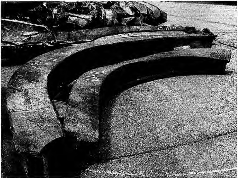
Figure 486. I-beams deformed in the wrong direction. This deformation is not consistent with overload. (NIST) http://wtc.nist.gov/images/DSCN0941_hires.jpg
