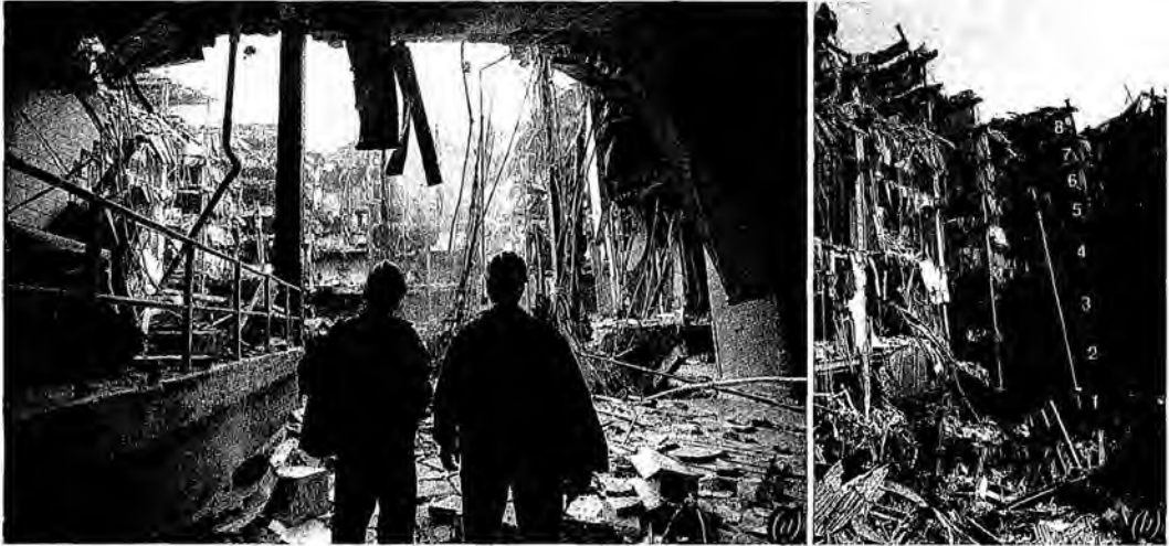
Figure 202. (9127/01) (a) Two people view the inside of WTC6. (b) Inside the 8-story WTC6 hole.
