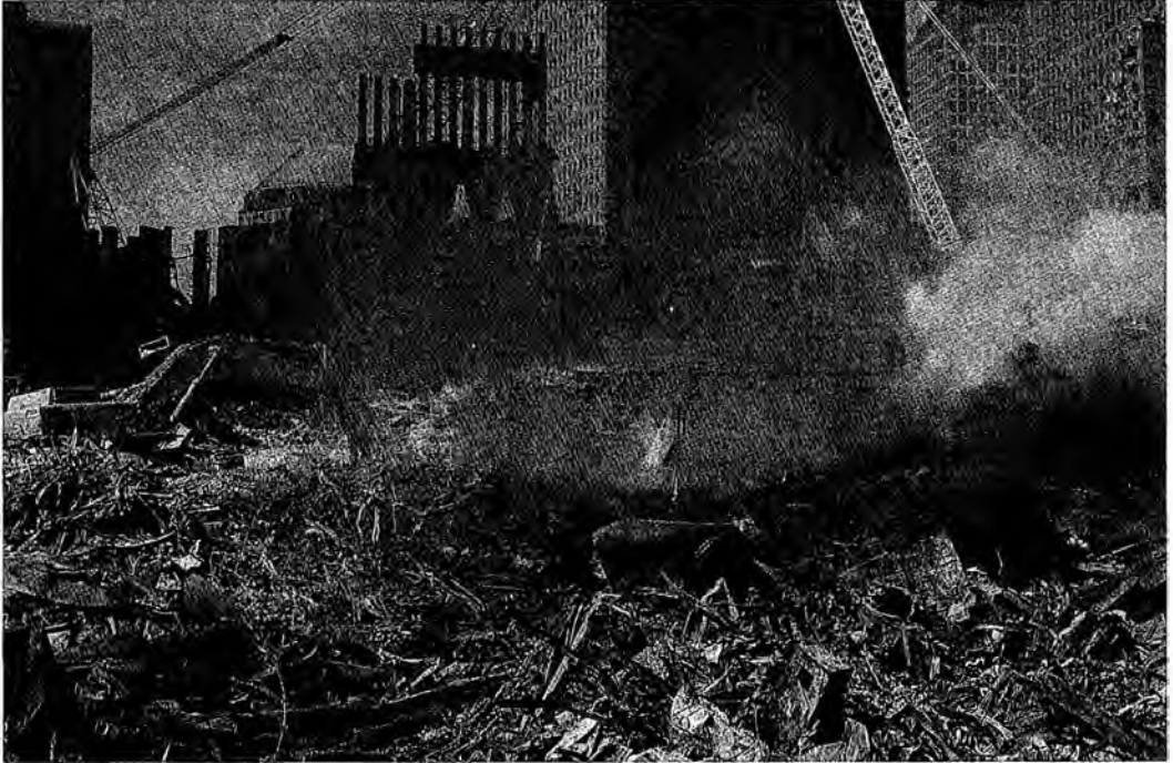
Figure 276. (10/13/01) Fire does not cause instant and uniform rust. (The orange fumes are probably from oxy fuel torch cutting.)
